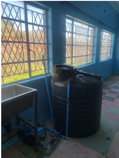
Figure 1: The connected tank behind the premises.
