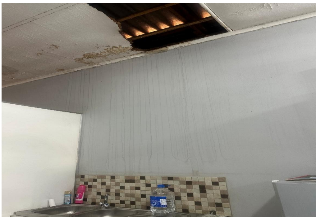
Image III showing gap in ceiling, water stains on wall and ceiling
