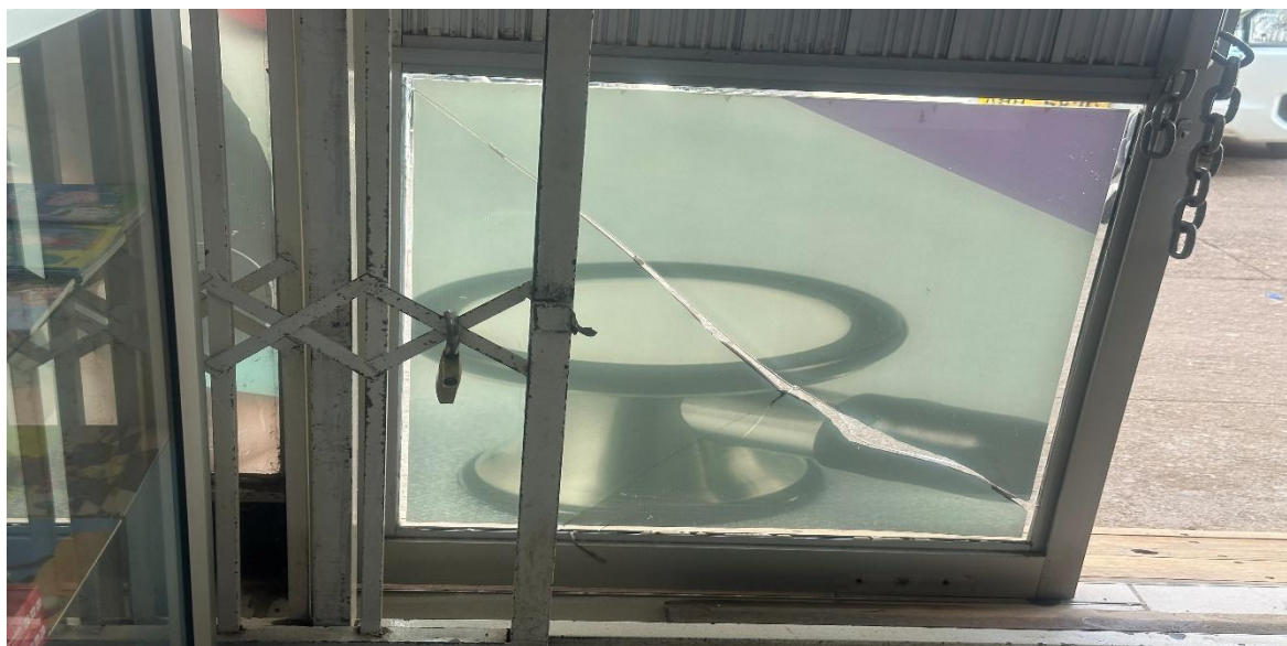
Image II showing cracked glass in front glass wall
